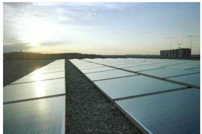
40 KW Solar photovoltaic system on a commercial building in Pittsburgh, PA, Installation and photo by Mountain Solar, Grass Valley, CA.
