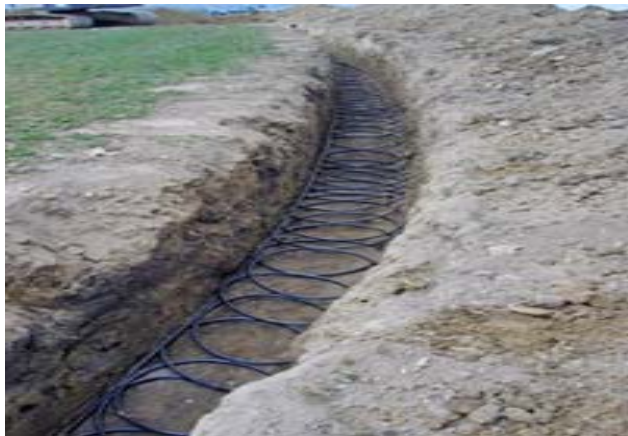
Geothermal heat pump being installed near Canandaigua, New York. Photo by RadiantMax.
