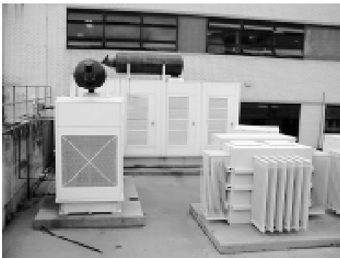
Diesel generators located behind the St. Paul Medical Center in Dallas
