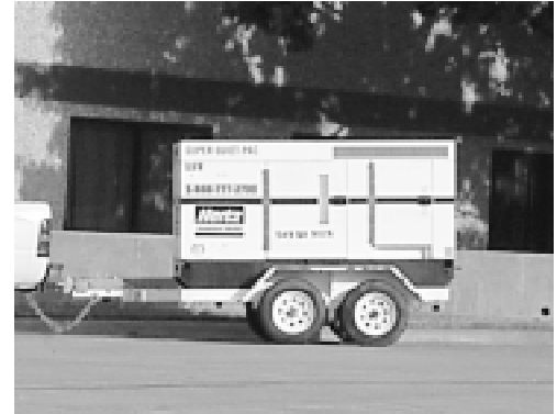
Portable 60 kW diesel generator located behind the Honeywell facility in Richardson
