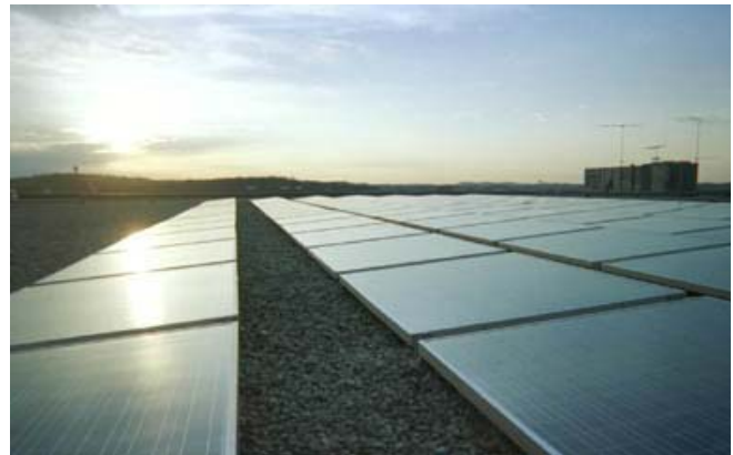
40 KW Solar photovoltaic system on a commercial building in Pittsburgh, PA, Installation by Mountain Solar, Grass Valley, CA.
