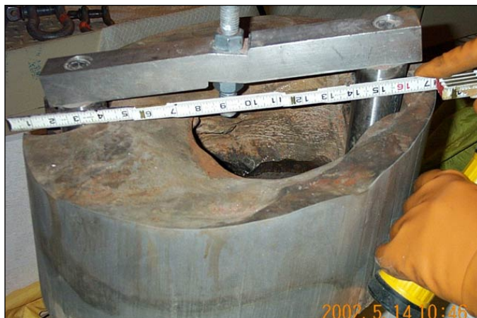
The hole in the head of the Davis-Besse reactor in Ohio.
