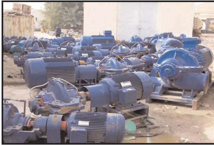
Idle water pumps outside of Hilla.
