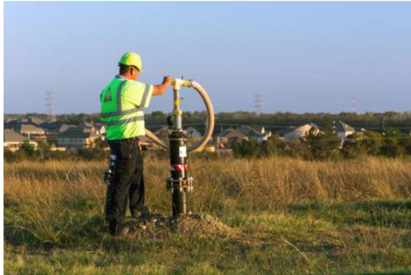
Among other changes, Republic Services Inc. said it is adding more gas wells like this one to contain odors from decomposing waste.
