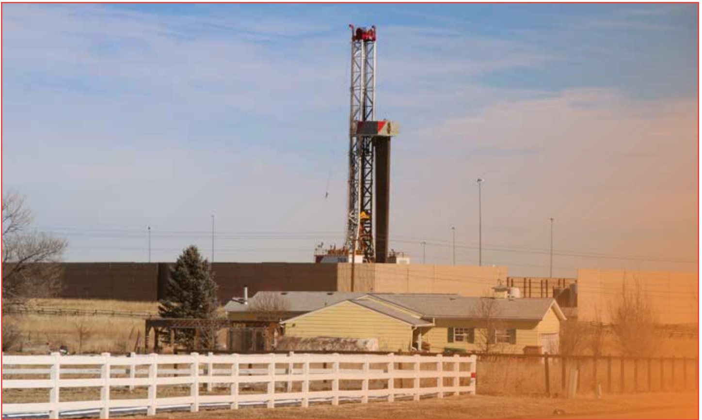
A Civitas drilling rig adjacent to residential communities in north of Denver. Photo: Andrew Klooster, Earthworks
