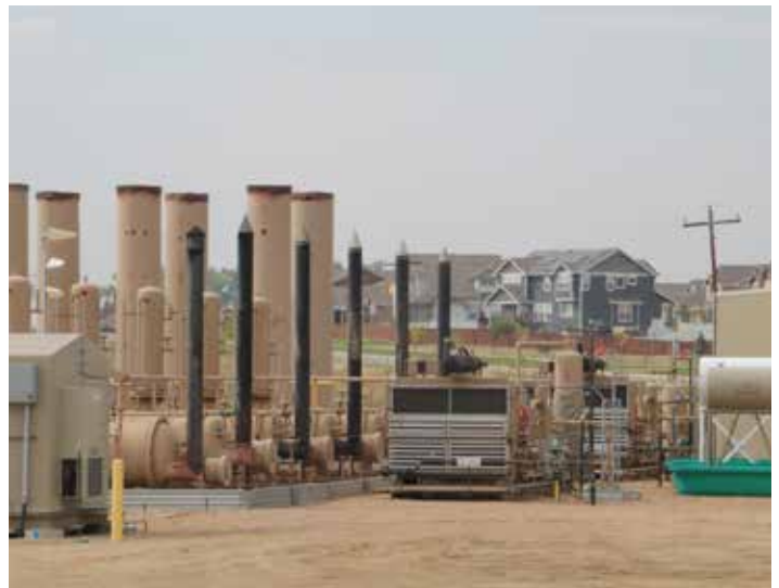
Oil and gas drilling equipment adjacent to homes and a high school in Severance CO. Photo: Earthworks
