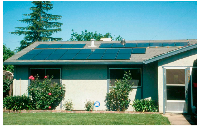
Grid-connected photovoltaic array
