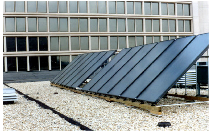
Domestic solar hot water heater
